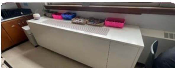
A unit ventilator with heating coils connected to the boilers
