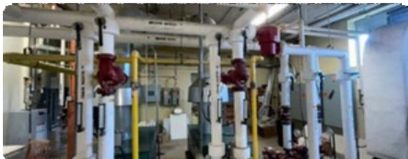
Natural gas fired atmospheric heating water boilers
