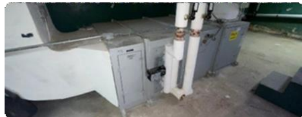
Air Handling Unit (AHU) with heating coils
