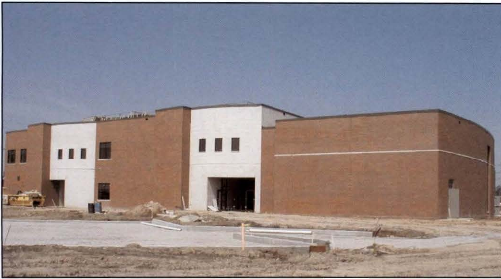
A view of the new 50,000-square-foot SIUE East St. Louis Center building from the northeast.
