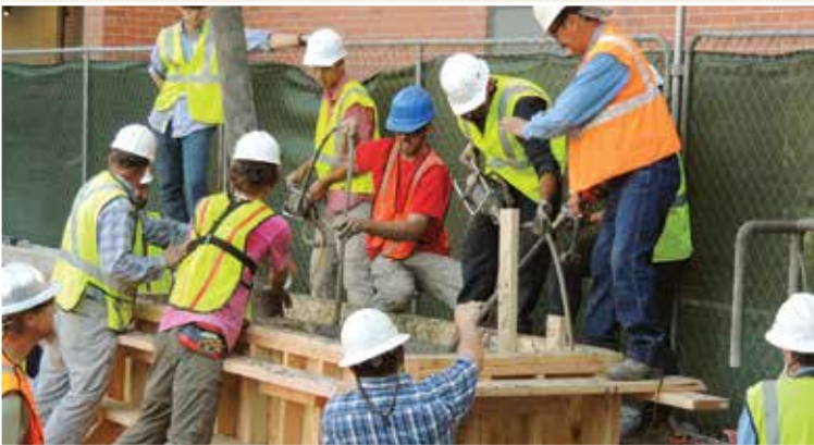
During the first large concrete pour, UAFM staff worked alongside the students, teaching them proper technique for placing and finishing concrete. During the second pour, students performed most of the labor with supervision by UAFM staff. During the third pour, the students worked with minimal supervision by UAFM staff. (Photo by Mark Marikos)
